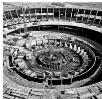
Figure 4. Zvartnots Airport in Yerevan. Foundations, structures of external radius. Photo of the late 1970s.
